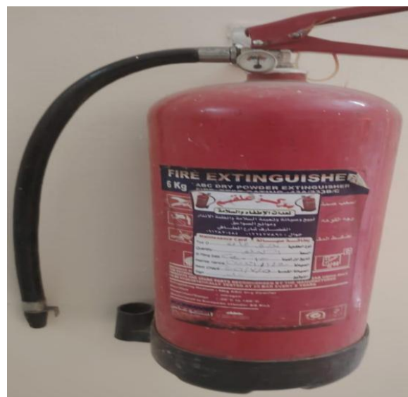
Figure 18/ 6 Kilo fire extinguisher
